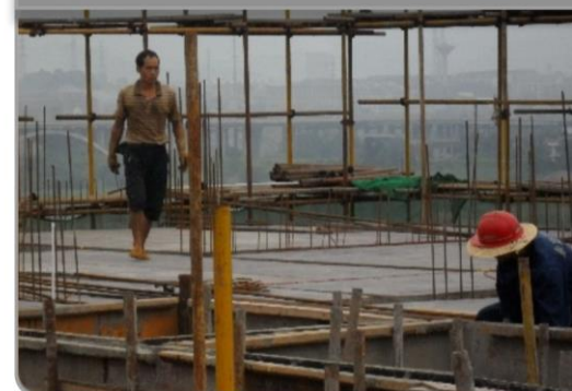
Safety problems occur frequently
