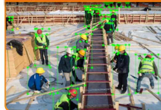
Automated safety monitoring system
